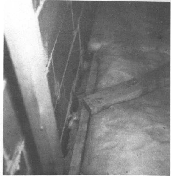
Gap at attic floor.
