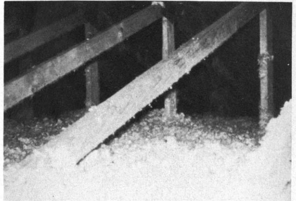
Blown fiberglass insulation lies on top of original batt insulation on attic floor, part of Princeton retrofit package A.
