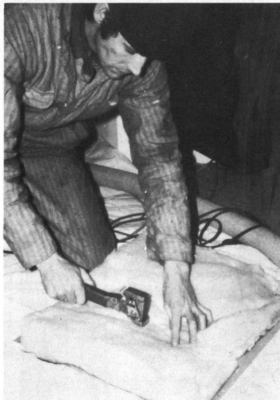
Insulation batt being stapled onto attic floor trap door, part of Princeton retrofit package A.
