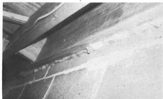
Plug of gap from basement by fiberglass, part of Princeton retrofit package B.
