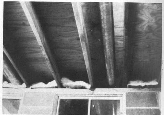
Ducts passing into living room overhang, casually insulated.
