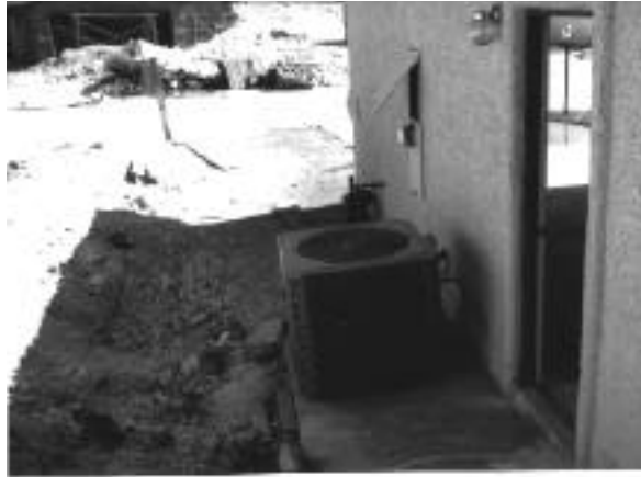
The placement of this air-conditioning unit in a location that provides afternoon shade will help to reduce the radiant heat gain in the outdoor coil during the hottest part of the day.
